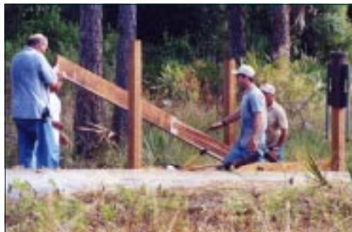
Ed and crew construct the final section of boardwalk by the wildlife crossing, above.
